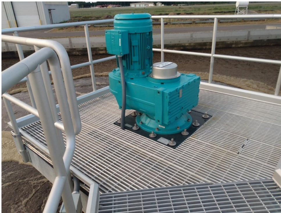
Aeration Weir Actuators
