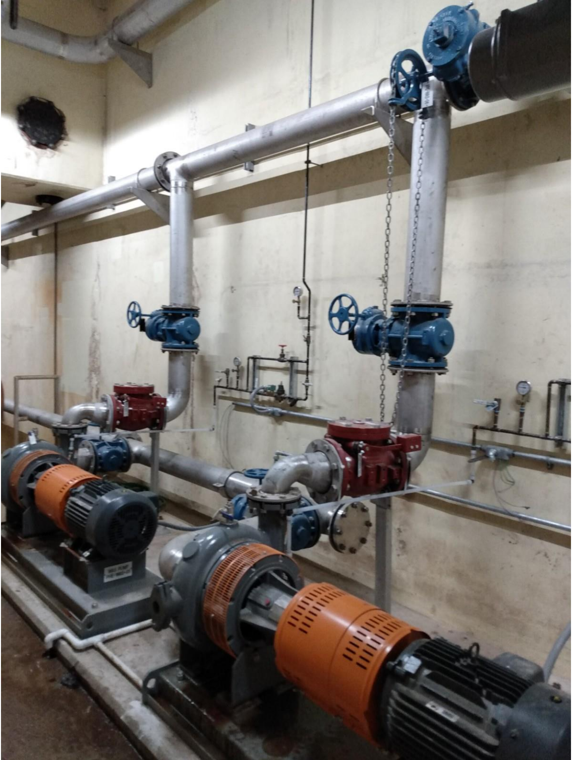
WS Pumps Valves
