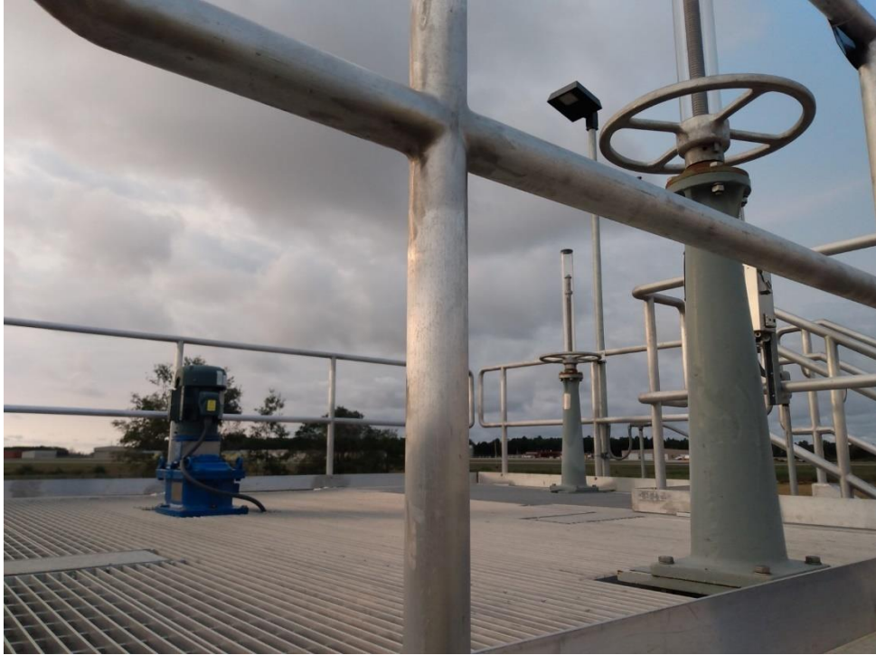
Rapid Mix Gates Motor
