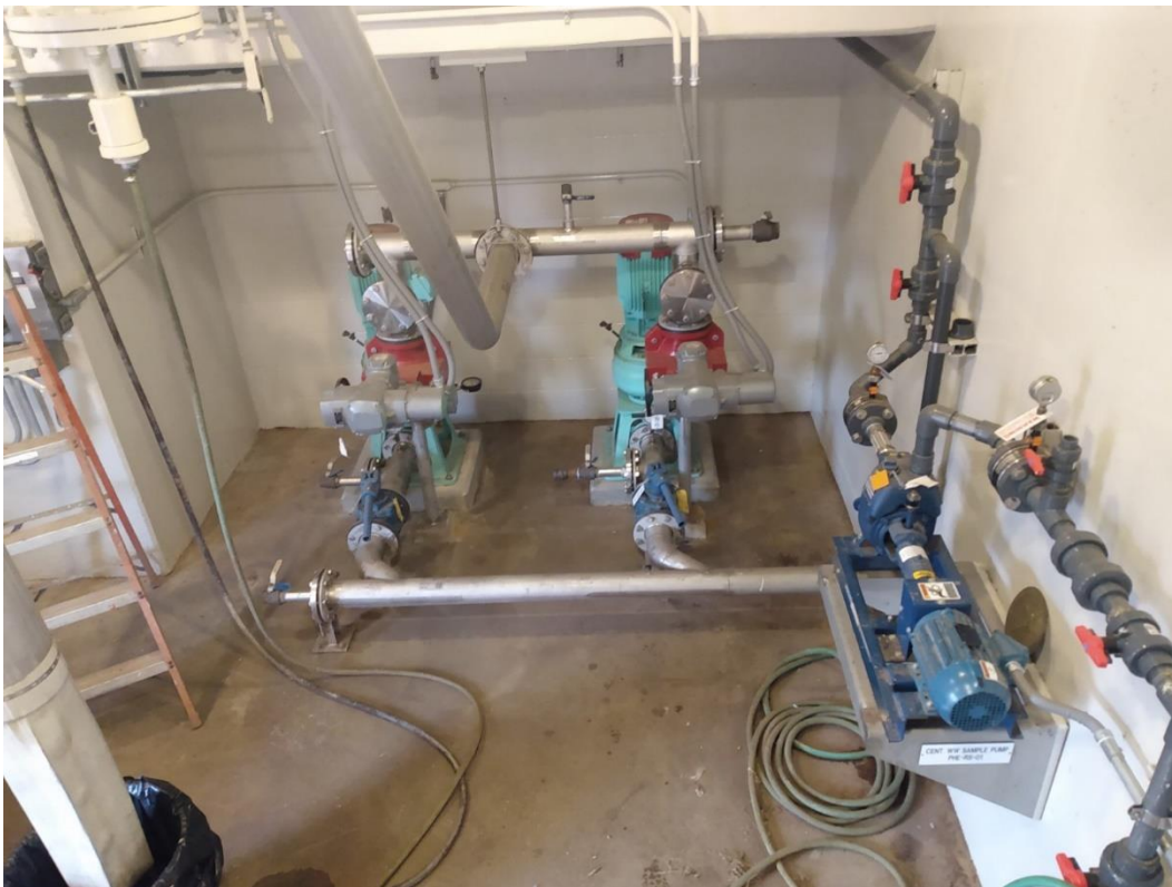
Grit Pumps Sampler
