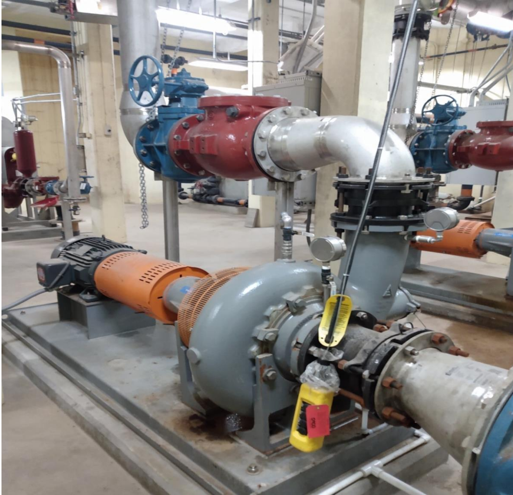
RAS Pumps Valves
