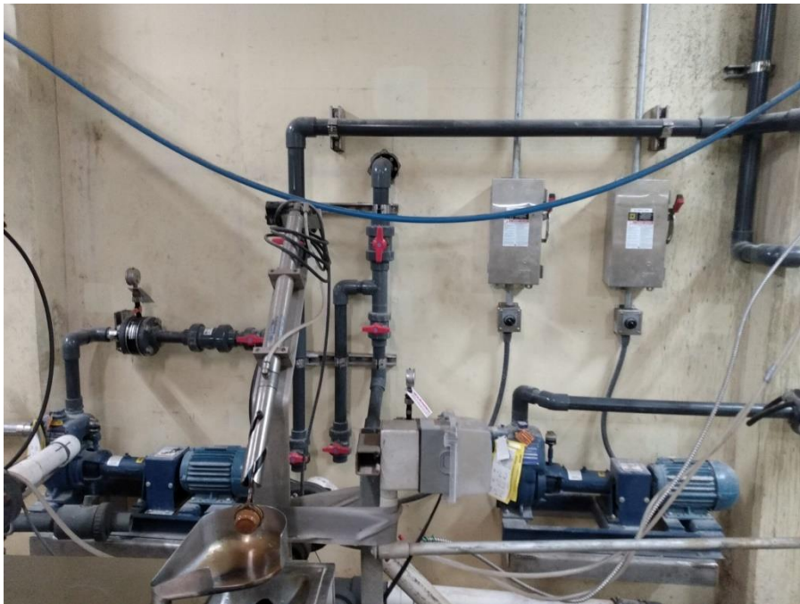
Secondary Sample Pumps
