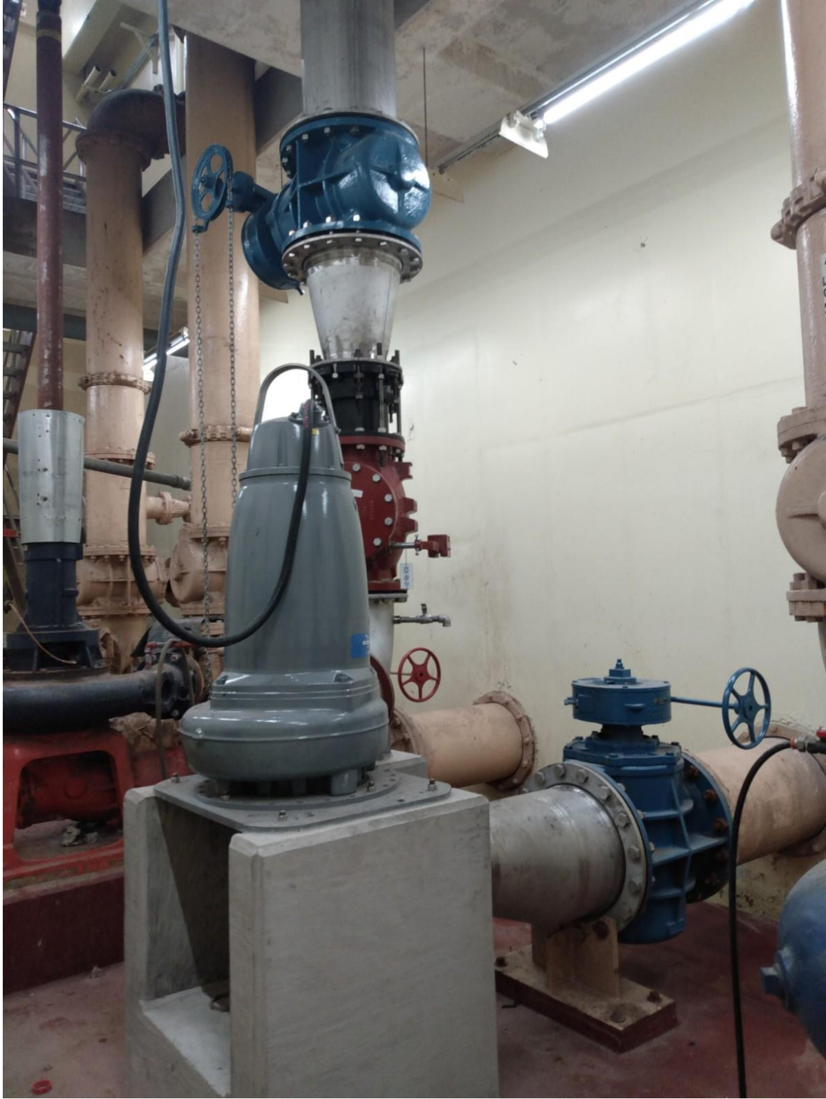
RAS Pump Valves
