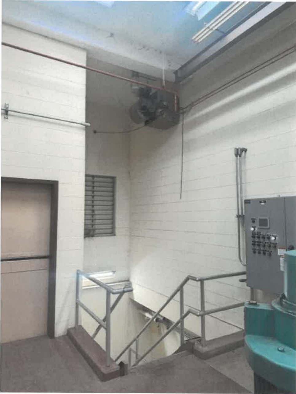
Figure 4 Bar Screen Heater with blower to heat room on the other side of wall. We may want to install a platform to work off below this unit.
