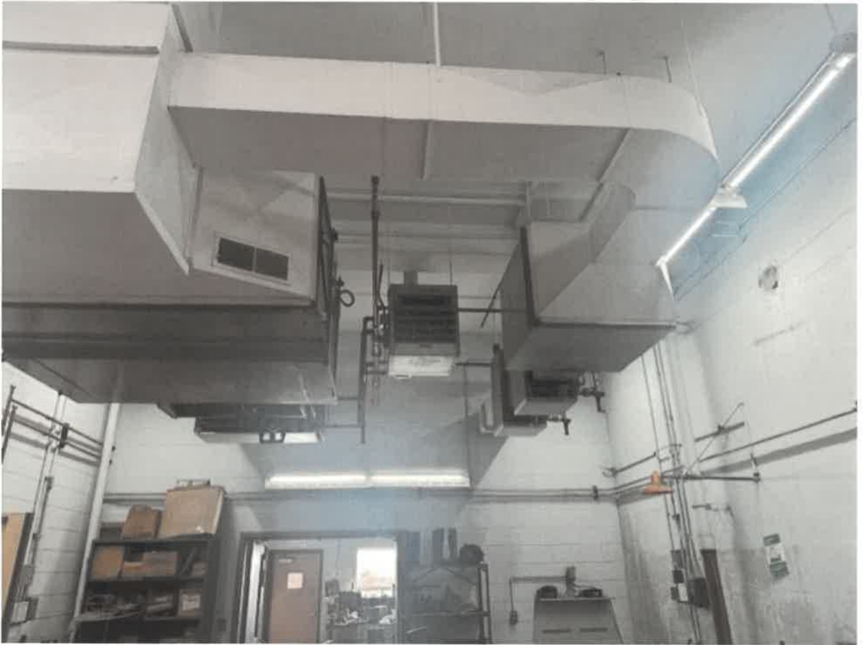
Figure 8 Headworks Garage Heater
