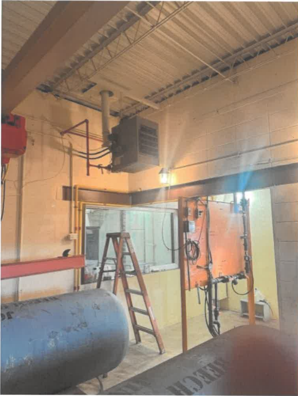
Figure 6 Cl2 room heater, may want a bigger unit heater to heat both rooms?
