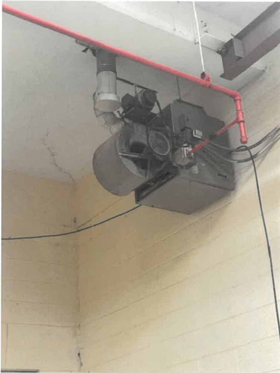
Figure 5 Bar Screen Room close up-- with blower.
