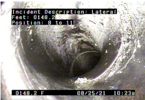
C - Crack @ 149.9 ft.
