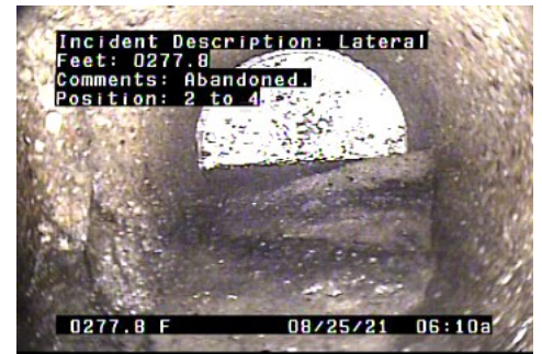
L - Lateral @ 277.8 ft. Abandoned.
