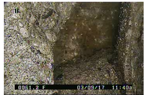
C - Crack @ 61.2 ft. wide crack possible exposed ground
