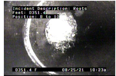
R - Roots @ 353.5 ft. Large root ball stopping camera. 90 feet of pipe has not been televised.
