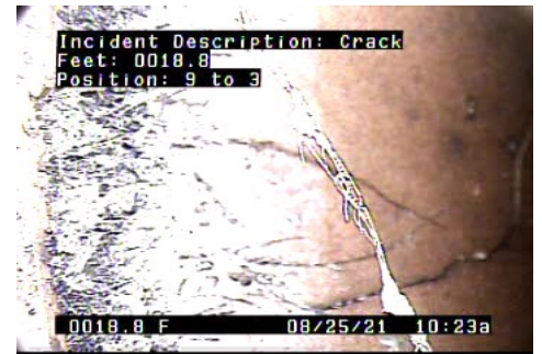
C - Crack @ 23.8 ft.
