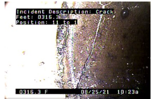
C - Crack @ 316.3 ft.
