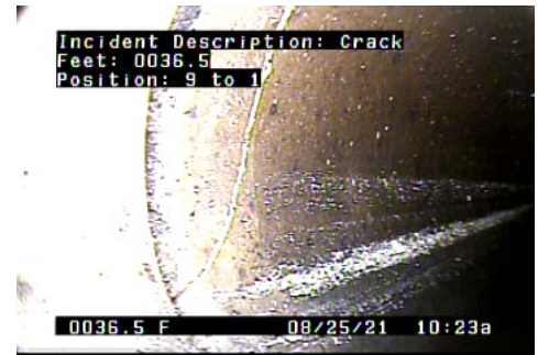
C - Crack @ 36.5 ft.
