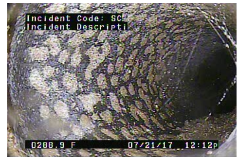
SC - Service Connection @ 288.9 ft.
