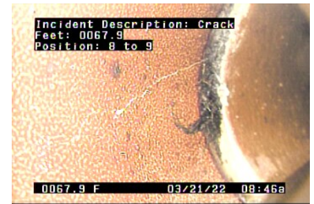
GO - General Observation @ 84.1 ft. Small bump in pipe with crack at the center.
