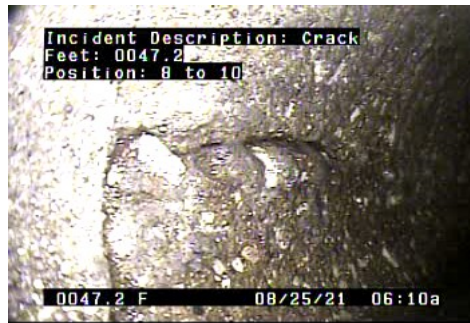
I - Infiltration @ 60.7 ft.
