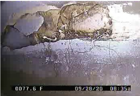
C - Crack @ 77.6 ft. Real Bad!
