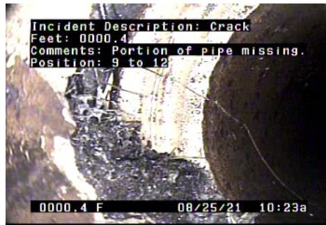
C - Crack @ 0.4 ft. Portion of pipe missing.
