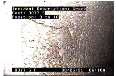
C - Crack @ 107.6 ft.
