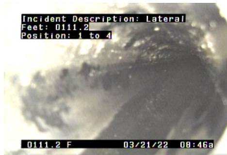
C - Crack @ 111.2 ft.
