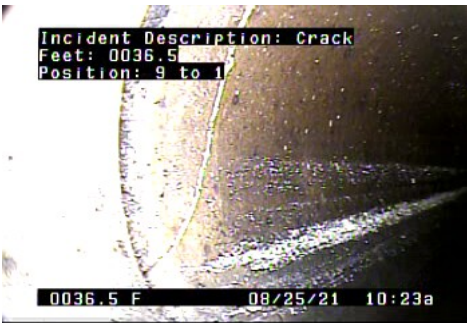
C - Crack @ 39.4 ft.
