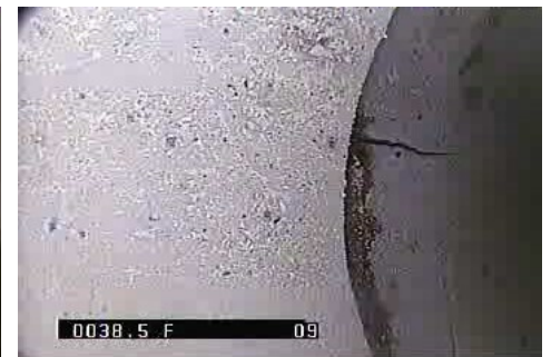
C - Crack @ 38.5 ft.
