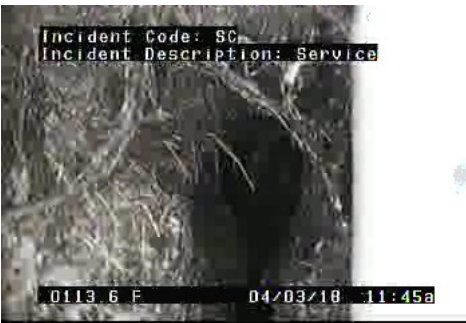
SC - Service Connection @ 113.6 ft. Roots in lateral
