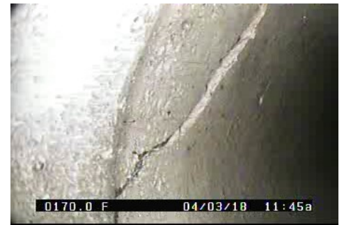
C - Crack @ 170.0 ft.
