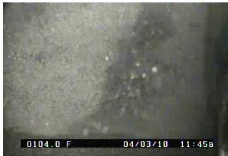
GO - General Observation @ 104.0 ft. Sand in bottom of the pipe
