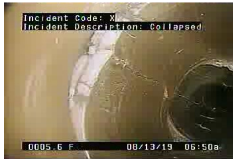
X - Collapsed @ 6.9 ft. Sewer collapsed
