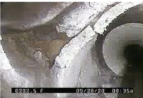
C - Crack @ 202.5 ft.
