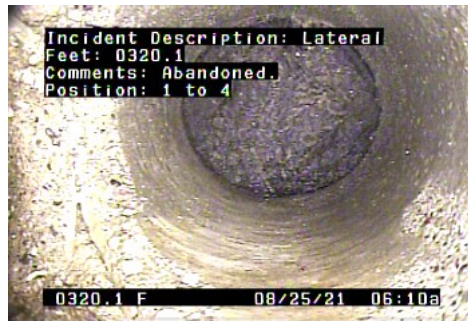
L - Lateral @ 320.1 ft. Abandoned.
