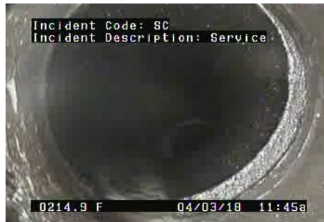
SC - Service Connection @ 214.9 ft.
