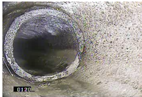
SC - Service Connection @ 120.1 ft.
