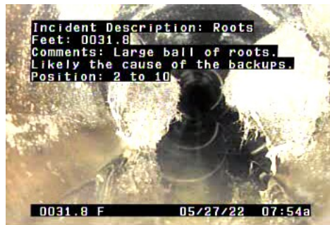
R - Roots @ 31.8 ft. Large ball of roots. Likely the cause of the backups.
