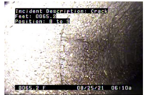
C - Crack @ 65.2 ft.
