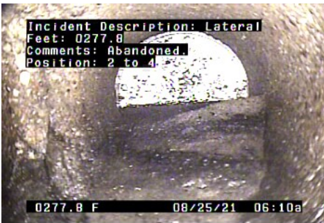
L - Lateral @ 317.0 ft. Abandoned.
