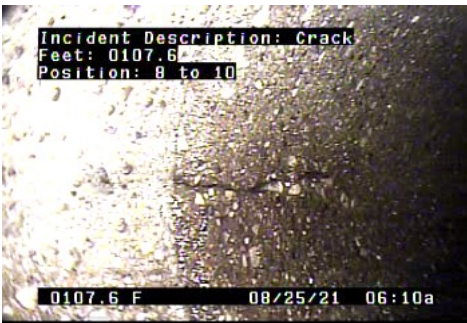
C - Crack @ 128.7 ft.
