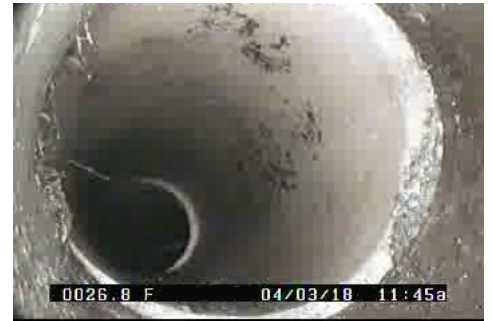
SC - Service Connection @ 26.8 ft.
