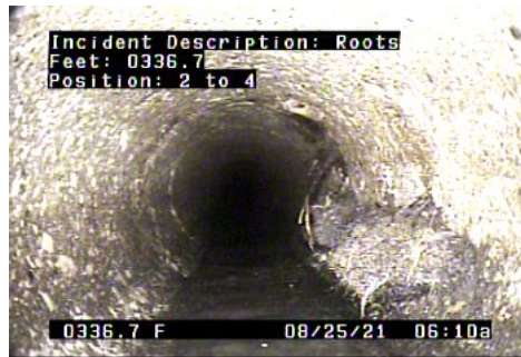
C - Crack @ 338.3 ft. Large root entering through pipe.
