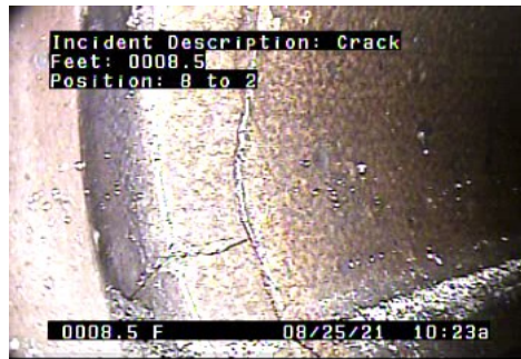
C - Crack @ 8.5 ft.
