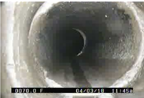
SC - Service Connection @ 70.0 ft.
