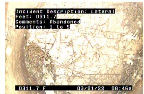
L - Lateral @ 311.7 ft. Abandoned
