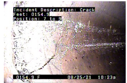
C - Crack @ 157.7 ft.
