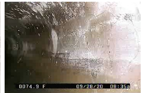
C - Crack @ 74.9 ft.
