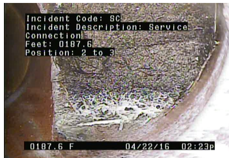
SC - Service Connection @ 187.6 ft.
