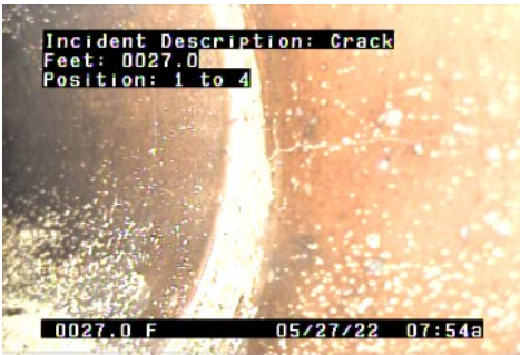
C - Crack @ 27.0 ft.
