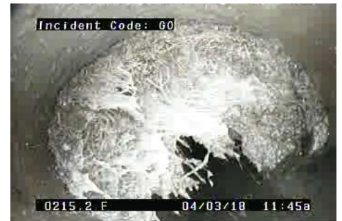
GO - General Observation @ 214.9 ft. Large amount of roots in the pipe.
