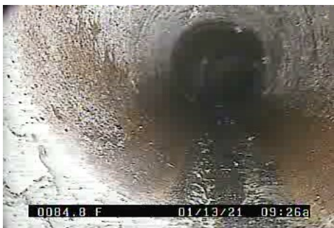
SC - Service Connection @ 84.8 ft.
