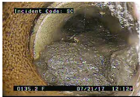
SC - Service Connection @ 135.2 ft.
