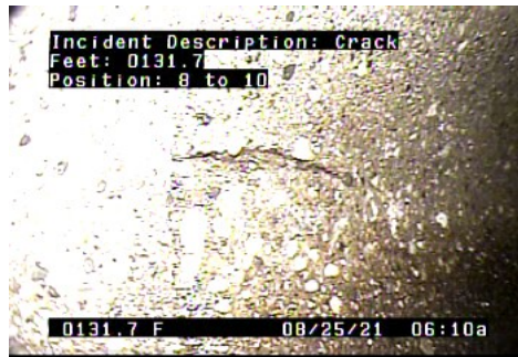
C - Crack @ 131.7 ft.
