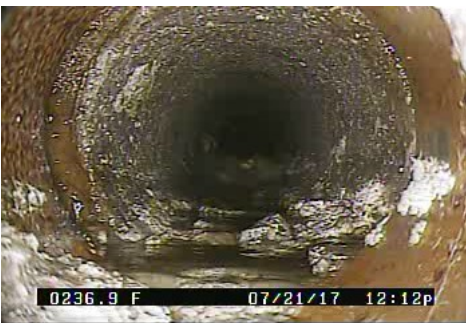
SC - Service Connection @ 236.9 ft.
