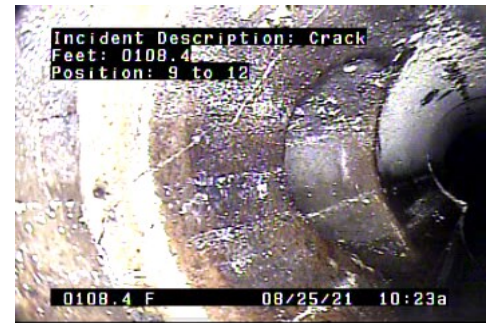
C - Crack @ 108.4 ft.
