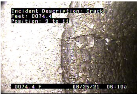
C - Crack @ 74.4 ft.
