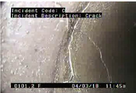
C - Crack @ 101.2 ft.
