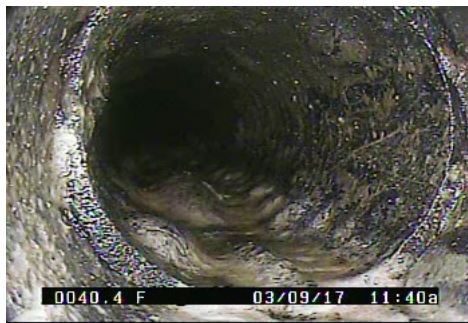
SC - Service Connection @ 40.4 ft.
