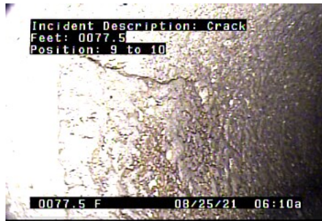
C - Crack @ 77.5 ft.
