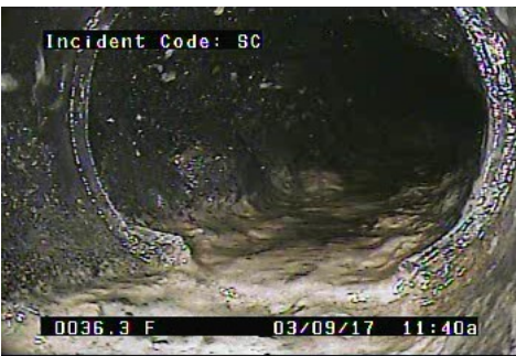
SC - Service Connection @ 36.3 ft.
