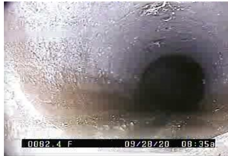
SC - Service Connection @ 82.4 ft.
