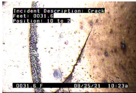
C - Crack @ 34.2 ft.
