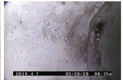
C - Crack @ 18.4 ft.
