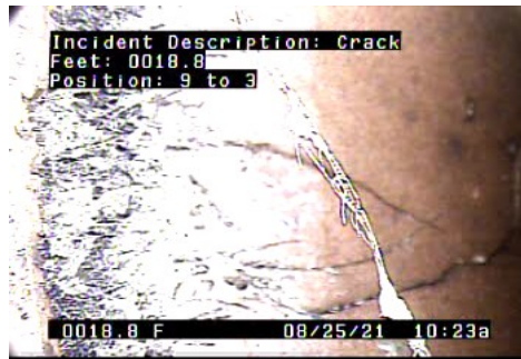
C - Crack @ 18.8 ft.
