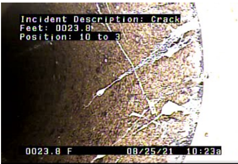
C - Crack @ 31.6 ft.
