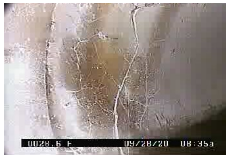
C - Crack @ 28.6 ft.
