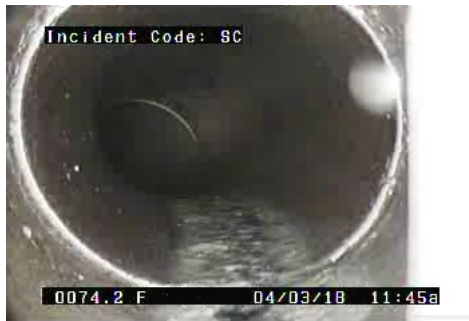
SC - Service Connection @ 74.2 ft.
