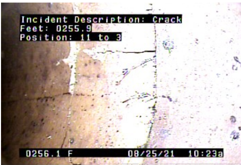
C - Crack @ 255.9 ft.
