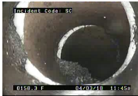
SC - Service Connection @ 158.3 ft.
