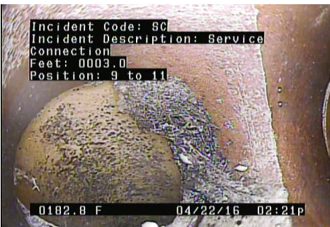
SC - Service Connection @ 3.0 ft.
