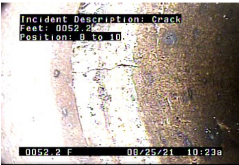
C - Crack @ 52.2 ft.
