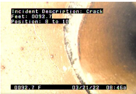
C - Crack @ 92.7 ft.
