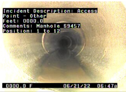
L - Lateral @ 8.0 ft. Abandoned
