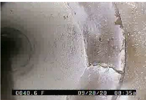
C - Crack @ 40.6 ft.
