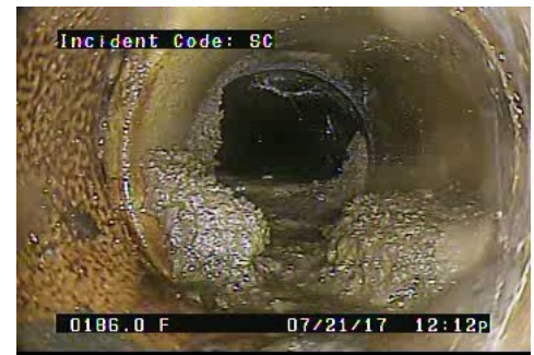
SC - Service Connection @ 186.0 ft.
