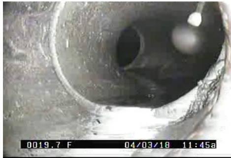
SC - Service Connection @ 19.7 ft.
