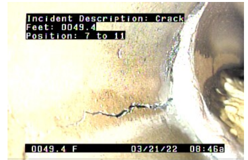
C - Crack @ 49.9 ft.
