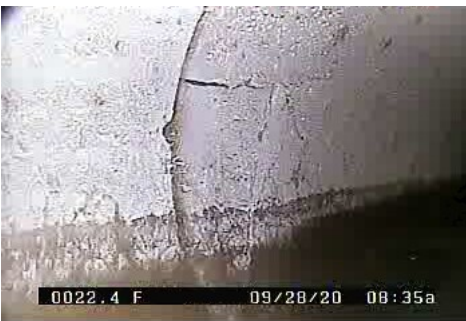
C - Crack @ 22.4 ft.
