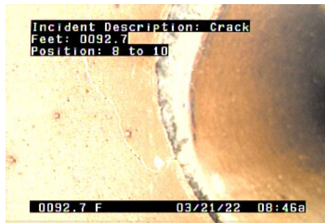
C - Crack @ 95.1 ft.
