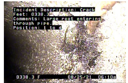
C - Crack @ 359.9 ft.
