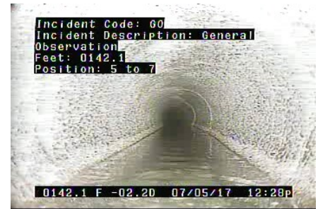
GO - General Observation @ 142.1 ft. Dip in pipe at about 140 feet, camera under water can't see.
