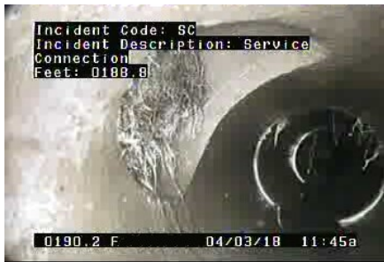
SC - Service Connection @ 188.8 ft. Roots in Lateral. Believe this is Mr. Lampi service connection.
