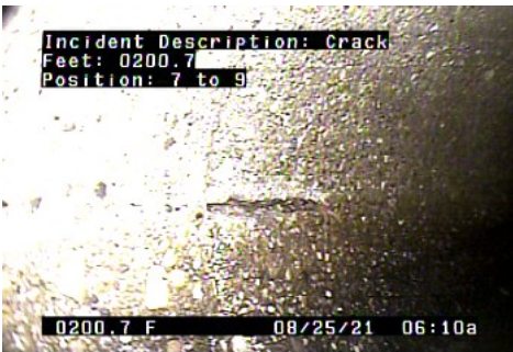
C - Crack @ 200.7 ft.
