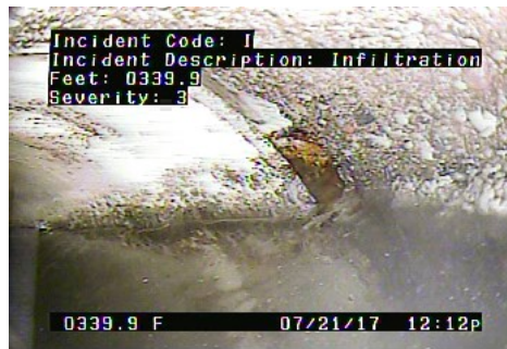
I - Infiltration @ 339.9 ft.
