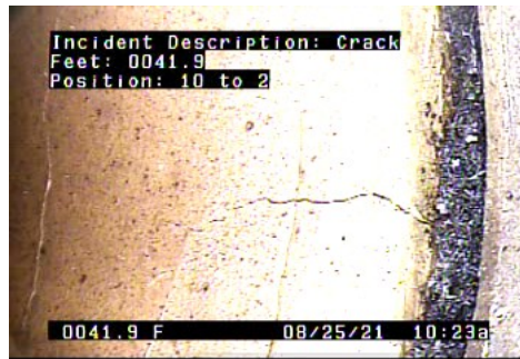
C - Crack @ 41.9 ft.
