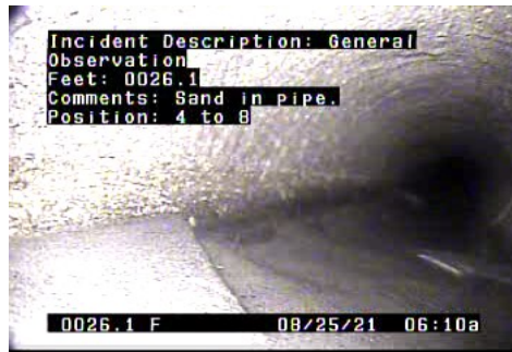
GO - General Observation @ 26.1 ft. Sand in pipe.
