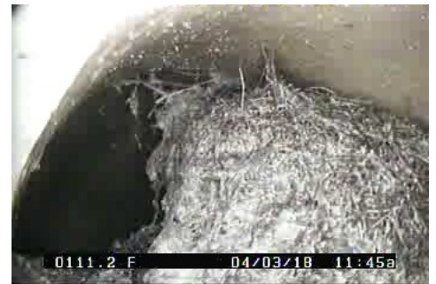
SC - Service Connection @ 111.2 ft. Roots in lateral
